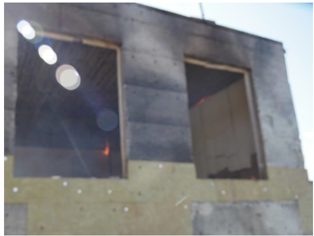
DLT ceiling and B302
