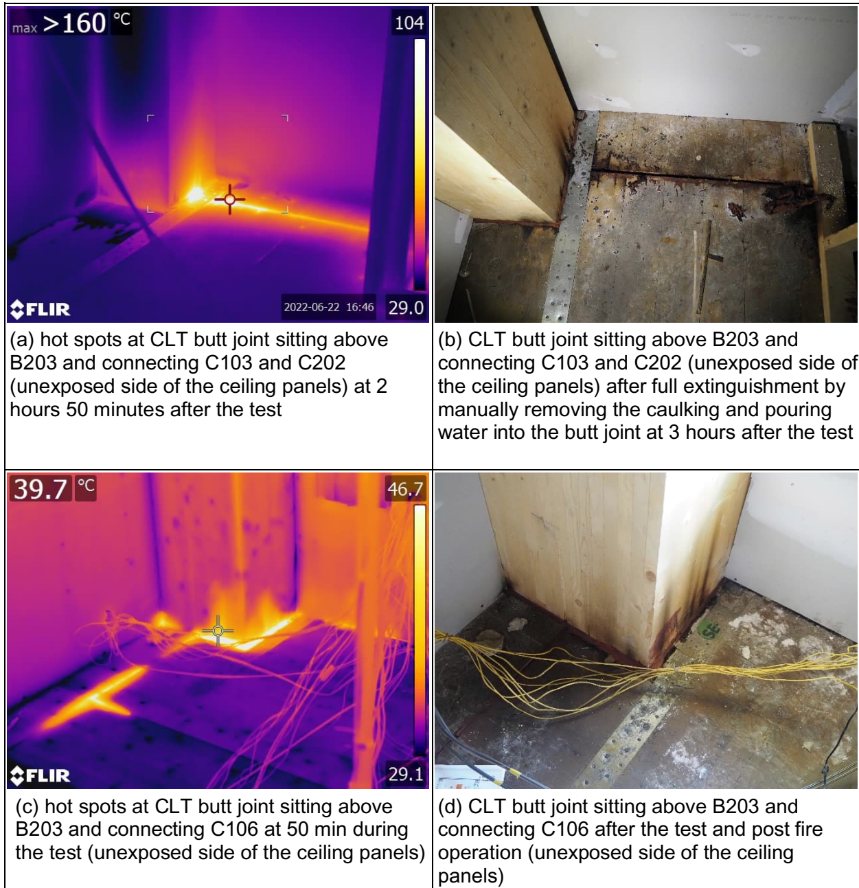
Figure 26. CLT-CLT butt joint and connection with columns on non-fire side in Test 5.
