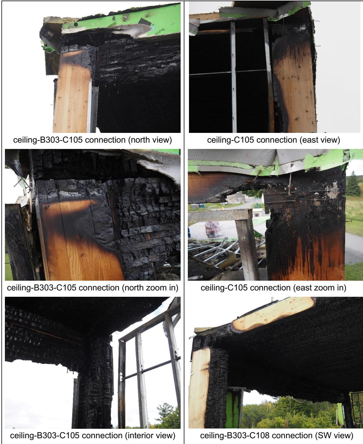
Figure 58. Charring on structural elements connected to beam B303 (Test 4).
