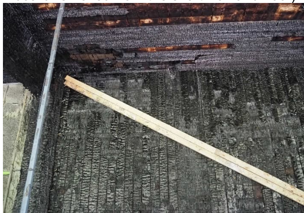
(c) hole in CLT floor-shaft junction (underside)
