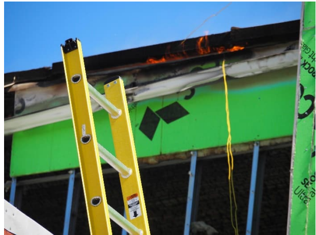
small flames in the DLT ceiling perimeter
