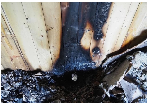
(a) hole in CLT floor-shaft junction (gypsum board removed from the shaft wall and floor)
