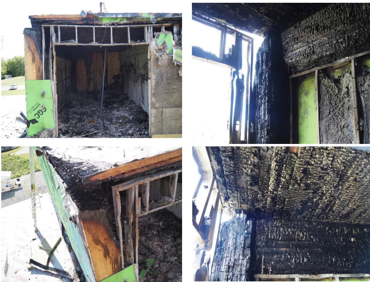
Figure 42. Charring near the B301-C201 beam-column-ceiling junction from Test 2.
